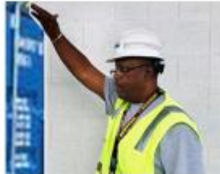
GANG IS PINNING or DE-PINNING: Keep hand on container OR arm outstretched in view of Crane Operator.
